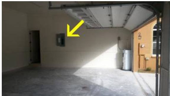
BRANCH PANEL DESCRIPTION: Siemens main panel, 200 Amp Maximum capacity, 200 Amp Main breaker installed.
